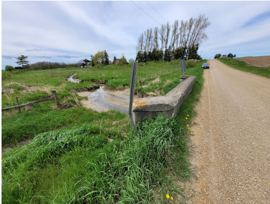
View of damaged southwest hazard sign.
