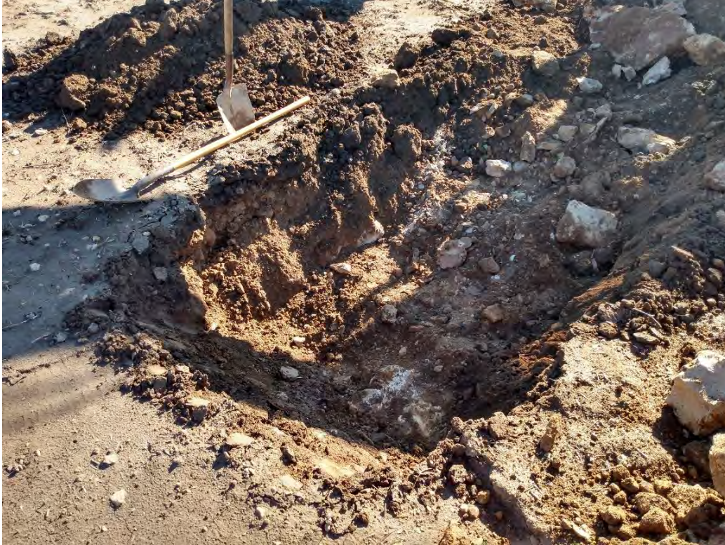
Photo 3: Exposed soil and bedrock in TP5 near the northwest corner of the Site (April 27, 2023).
