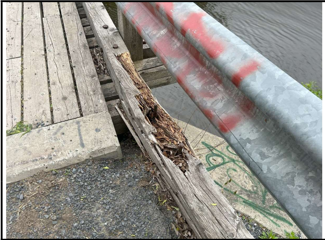
Photo 11 Severe weathering and rot on timber at west curb
