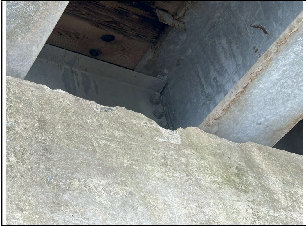
Photo 17 Spalls at top part of abutment wall
