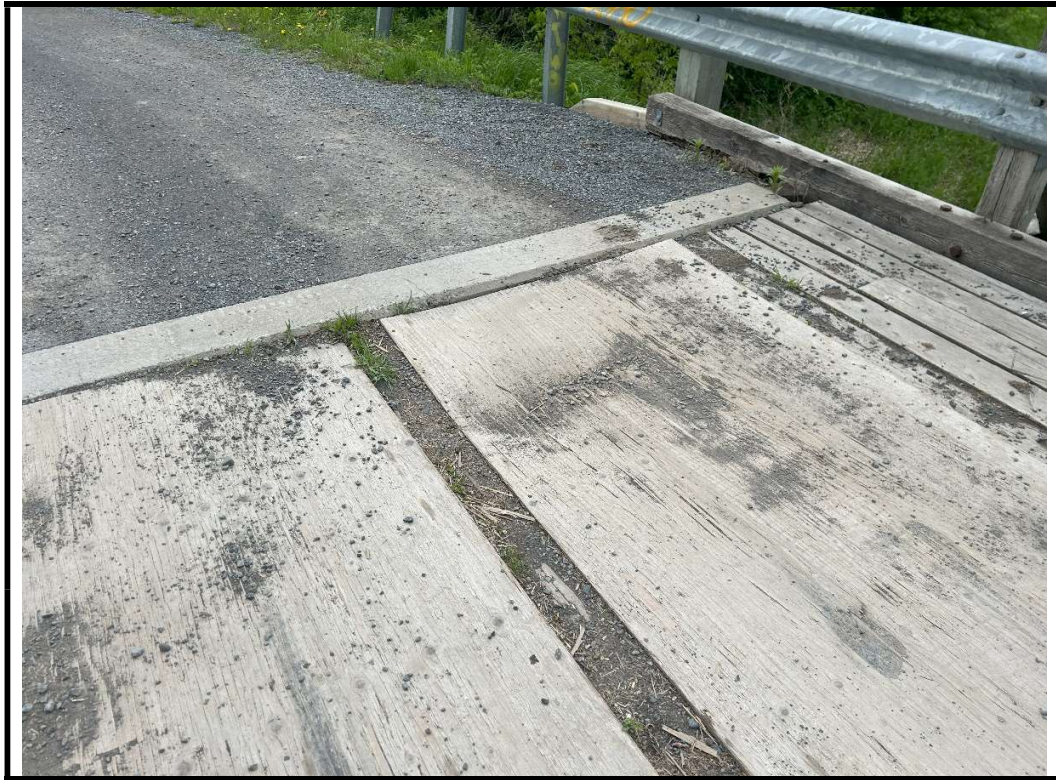
Photo 9 Severe depression at south end of deck
