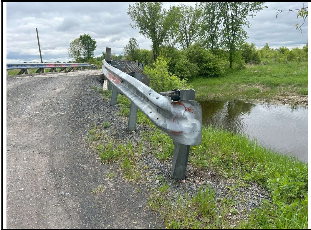
Photo 7 Collision damage at northwest railing system
