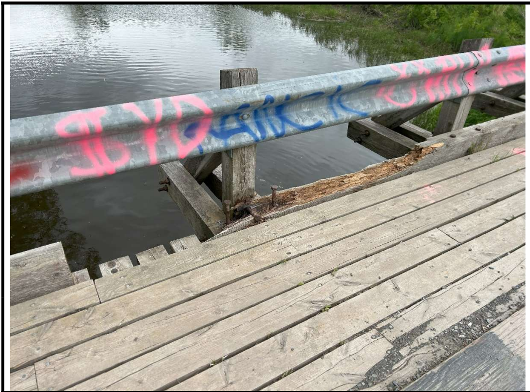
Photo 12 Severe weathering and section loss on timber at east curb
