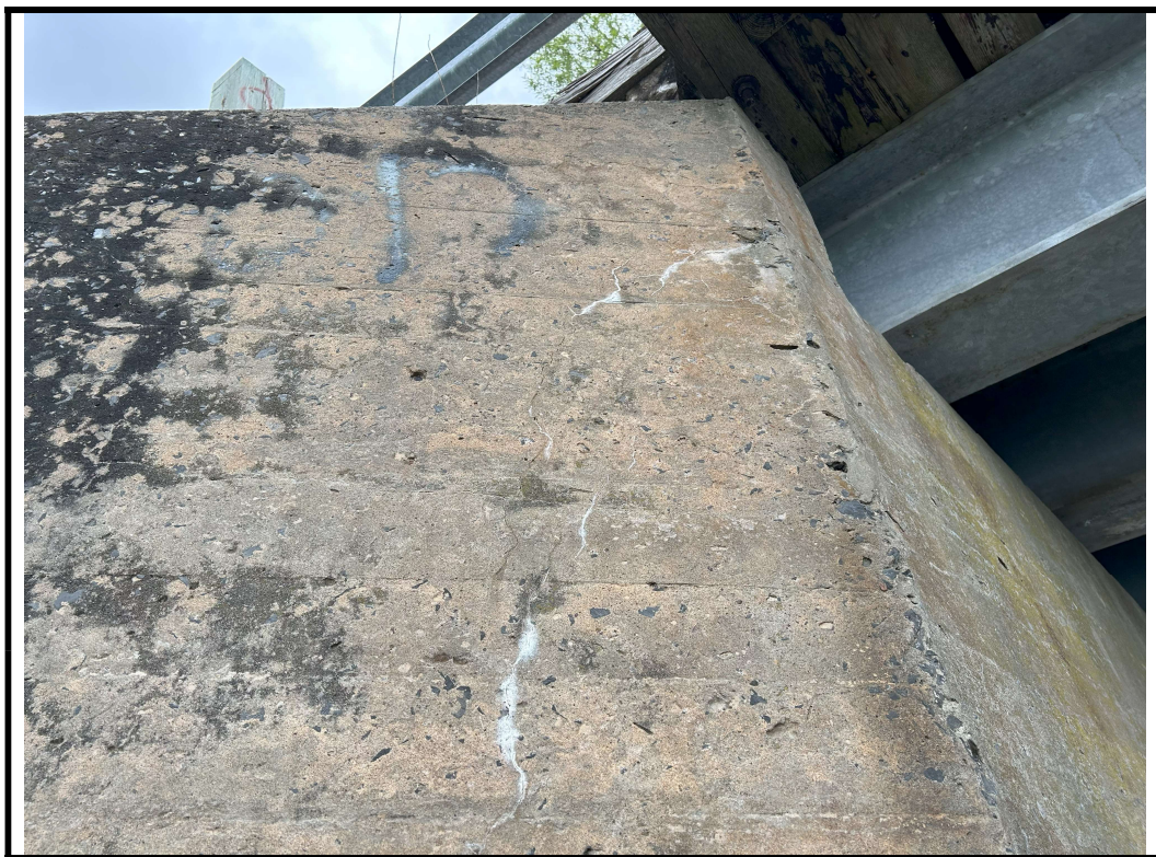
Photo 16 Narrow cracks with efflorescence at northwest wingwall
