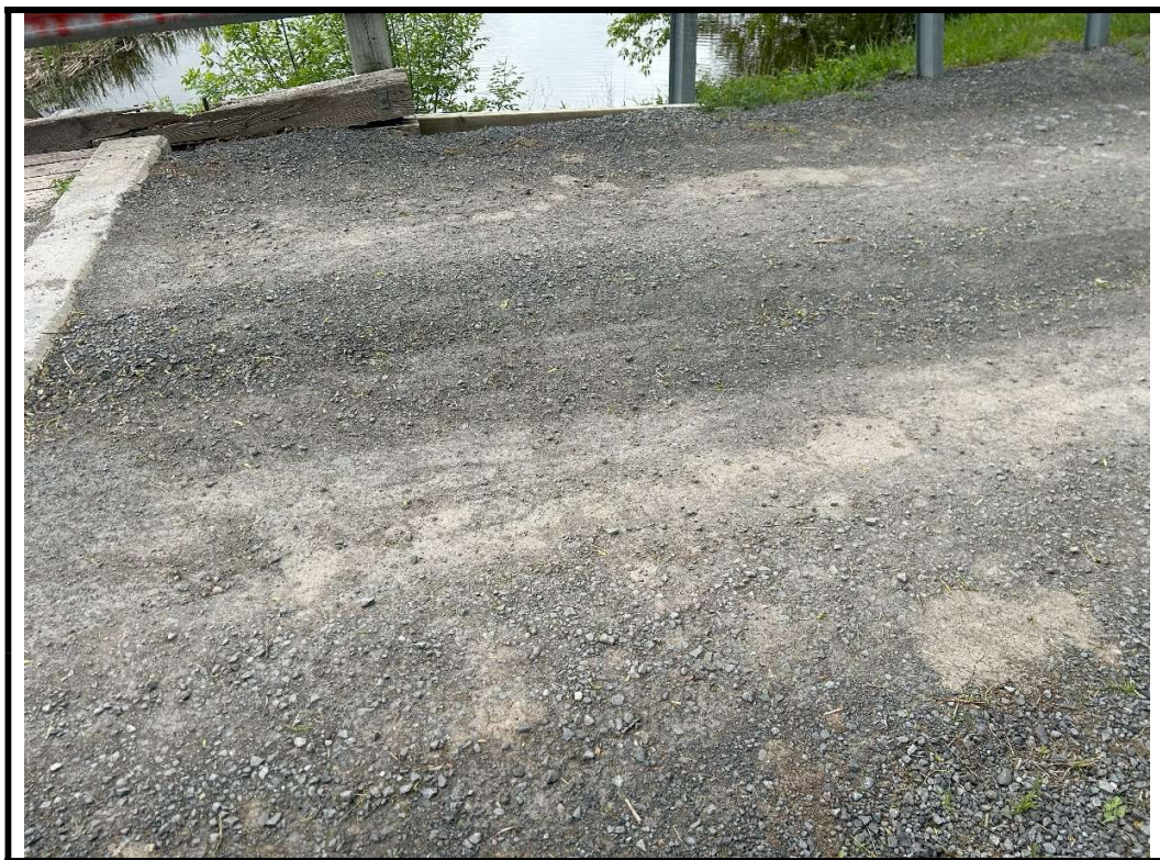
Photo 8 Depression at north approach wearing surface
