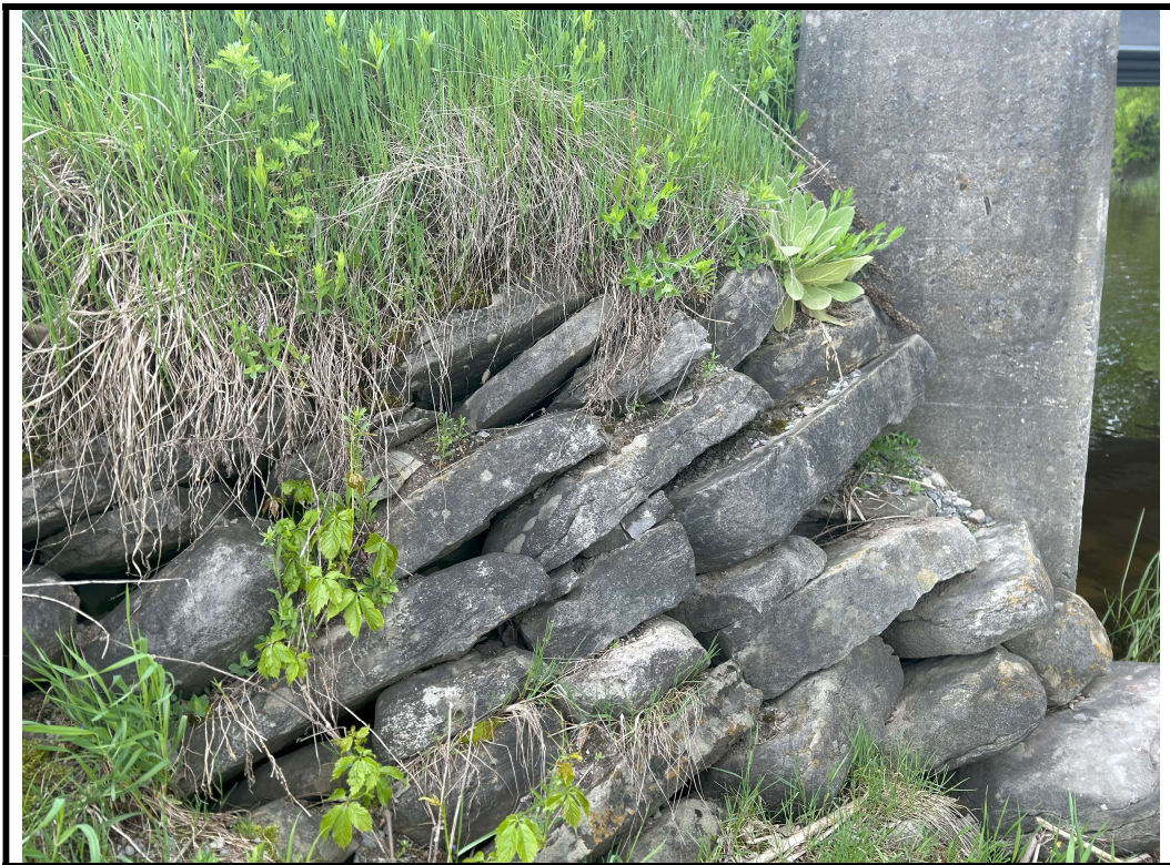
Photo 18 Leaning rock slope protection at southeast embankment
