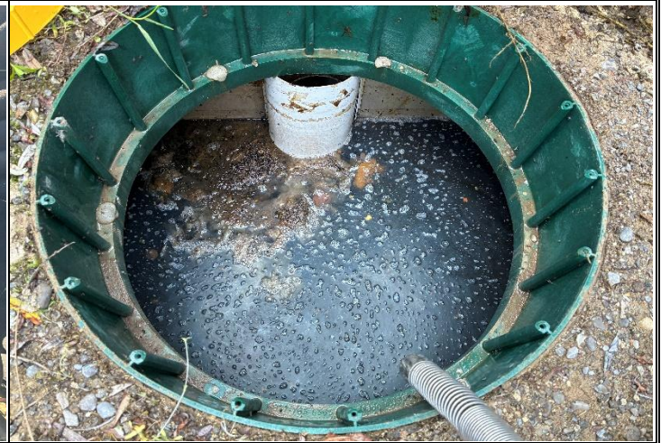
2. Septic tank inlet compartment
