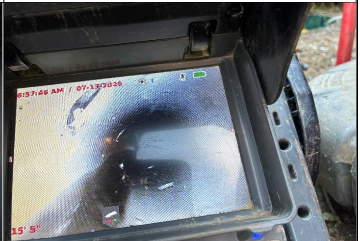
10. Interior of perforated distribution lateral
