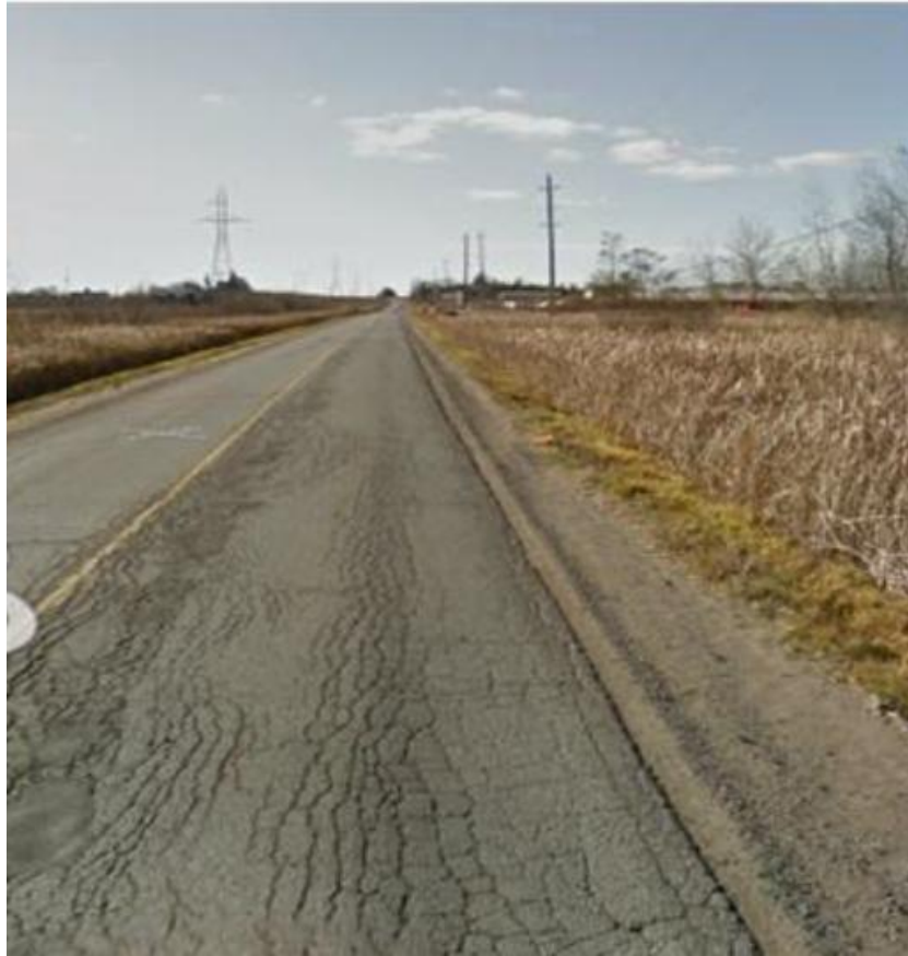
Figure 84 Road Surface in Poor Condition Example
